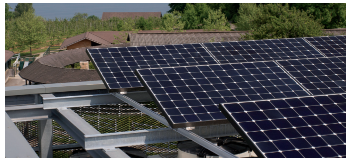
Solar panels on the roof of the building have a nominal electrical power of 38 kW.
